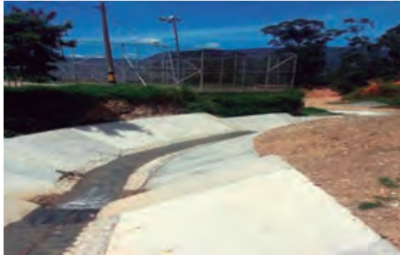
Construction of water works and first canalization stage of Zanjon del Alto, Peladeros and Sesteaderos streams.
